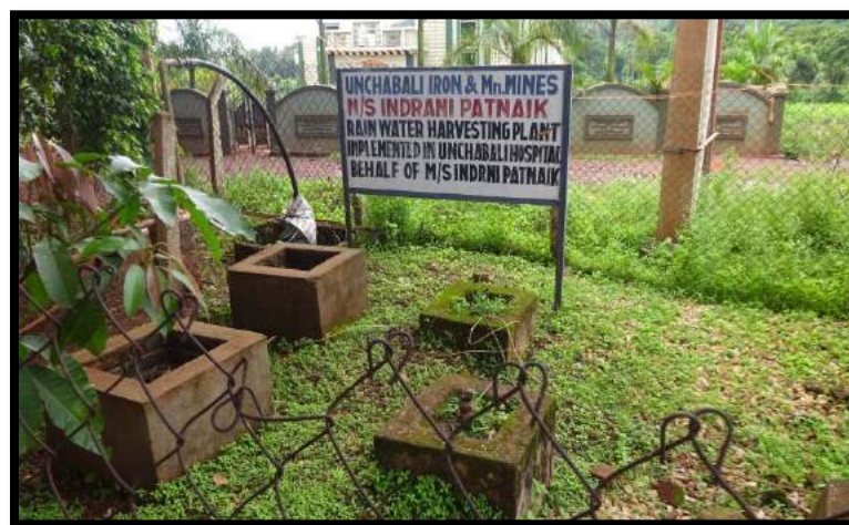
PHOTO SHOWING ROOF RAIN WATER HARVESTING SYSTEMS AT MINES & UNCHABALI DISPENSARY
