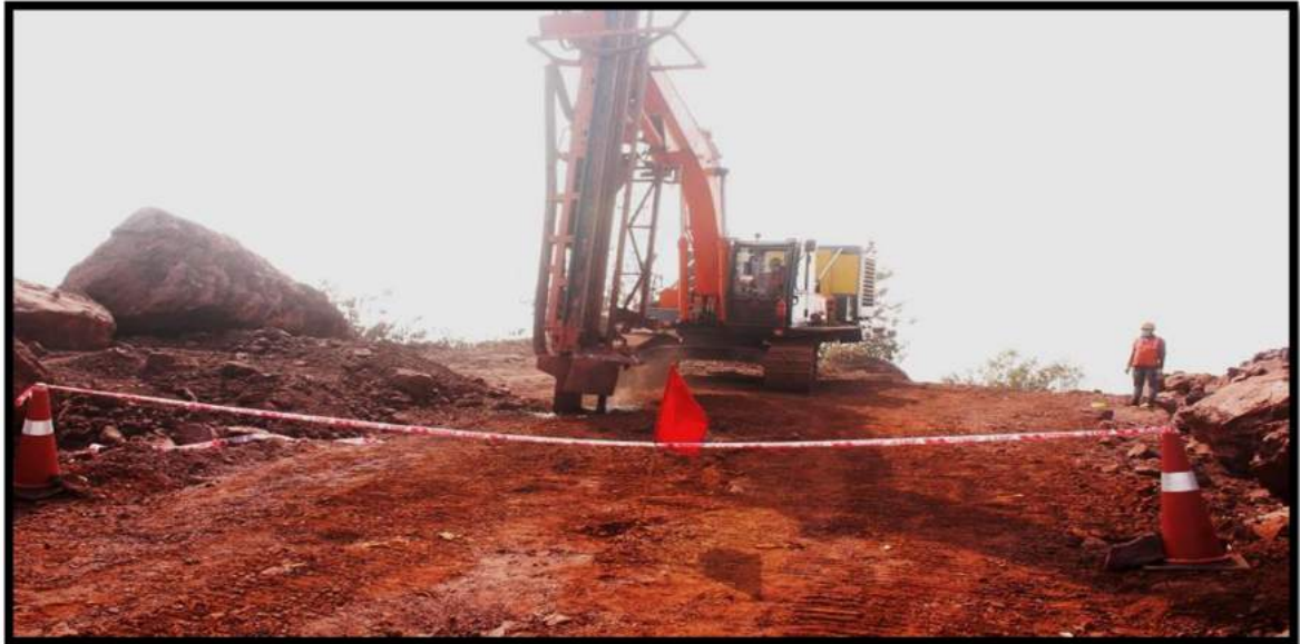
Photo Showing Excavated Mounted Drilling Machine equipped with dust extractor & wet drilling mechanism
