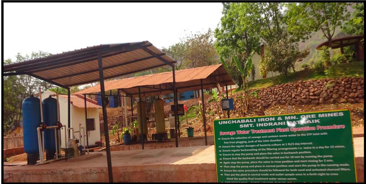
PHOTO SHOWING THE NEW STP INSTALLED AT CAMP FOR THE WATER TREATMENT
